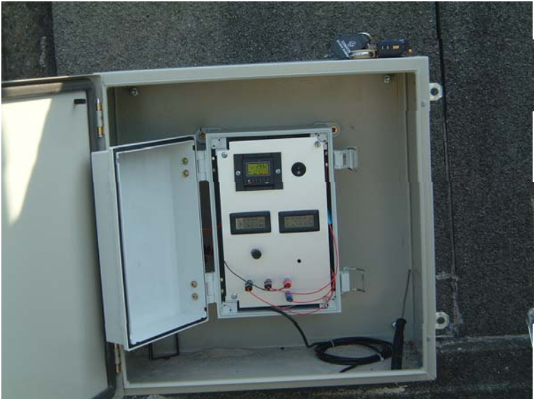
Automated monitoring box
