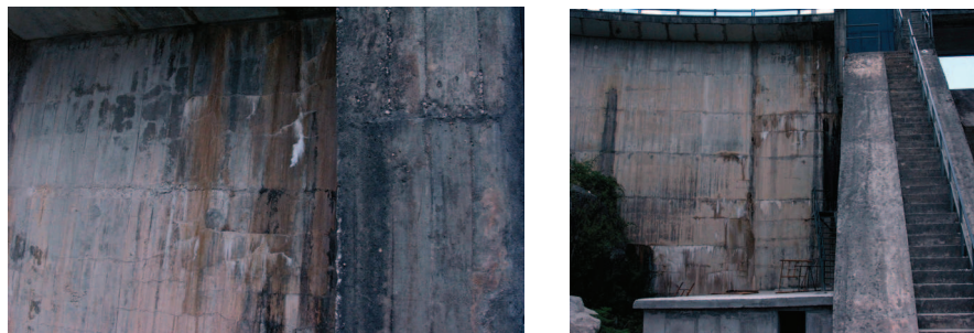
Figure 2: Horizontal cracks and map cracking in the right buttress and in the right arch.
